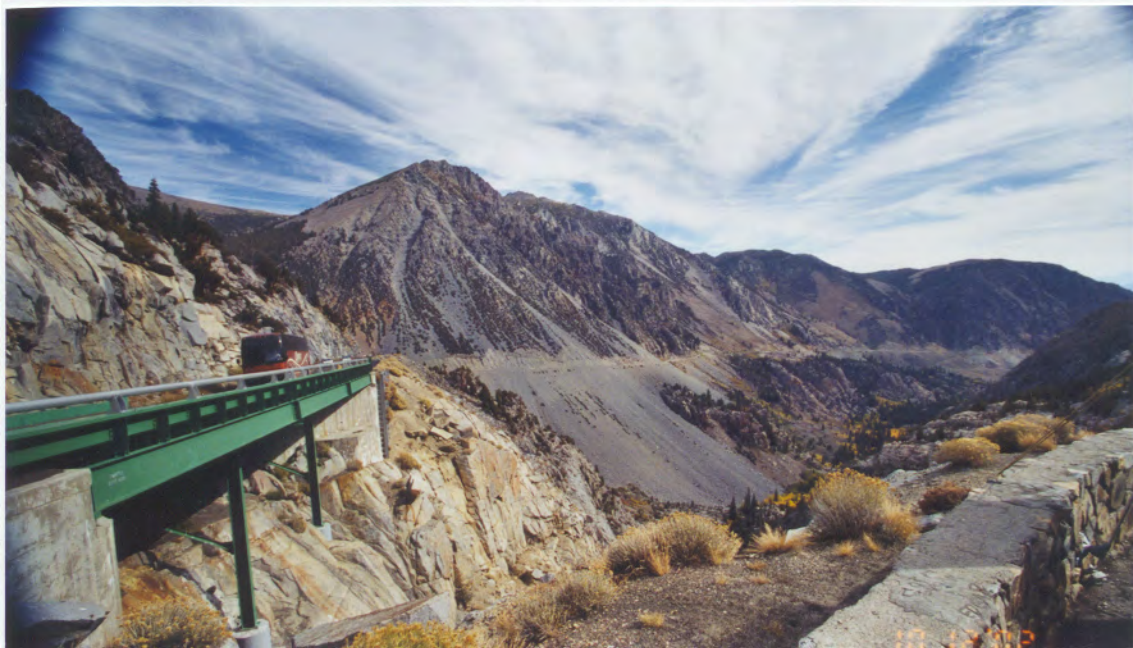
Sidehill viaduct just down grade from Dodge Point & our plaque. Lee Vining Peak beyond & Lee Vining Creek at right.
