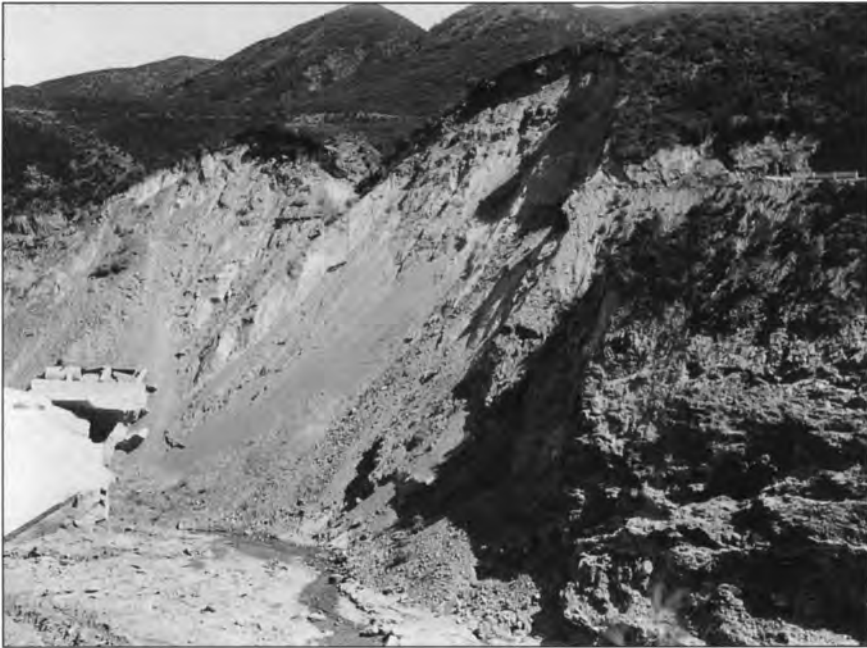
Figure 15 (upper) - View looking southeast, at east abutment slide scar, from position of Edison power poles, across canyon, after the failure. The enormity of the slide can be vividly appreciated, with a mass of well over 500,000 cubic yards.
