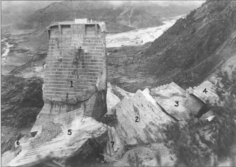
Figure 23 - Photo looking upstream showing the final resting positions of the east abutment and main section blocks. Note the schist detritus left upon Blocks 4 and 5, as well as the position of Block 7[41], behind Block 5. The oakum patch of the crack in Block 5 is also very apparent. Blocks 2/3/4 separated very late in the failure sequence, when much less water was available to dislodge them (they toppled upstream). Photo from University of California Water Resources Center Archives.
