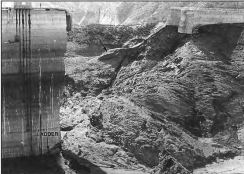
Figure 26 (lower) - Detail of failed west abutment, looking downstream, with people circled for scale. Only a portion of the sidecast fill for the construction road was excavated by the outpouring water (arrow), with scrub brush left upon the cut slope side down to elevation 1,775, 60 feet below the reservoir level. Photo by permission of Ventura County Museum of History & Art.
