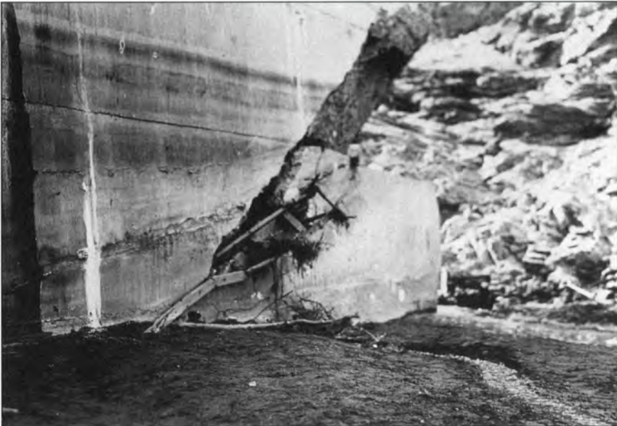
Figure 24 - Photo showing the upstream gage attendant's ladder wedged into a major crack at the west upstream heel of Block 1. This was often referred to as "Grunsky's ladder," because engineer C.E. Grunsky made its discovery after the reservoir's water had receded (the ladder was underwater for several days after the failure). Block 1 would have to have tilted at least 12 inches to swallow up the ladder, which was 18 inches wide. There is little doubt, therefore, that the upstream heel of the dam's central section was in tension and that, at some point, either before or during the failure sequence, full hydrostatic pressures must have acted upon the block's interior, significantly negating its effective dead load. Photo from Huber Collection, University of California Water Resources Center Archives.
