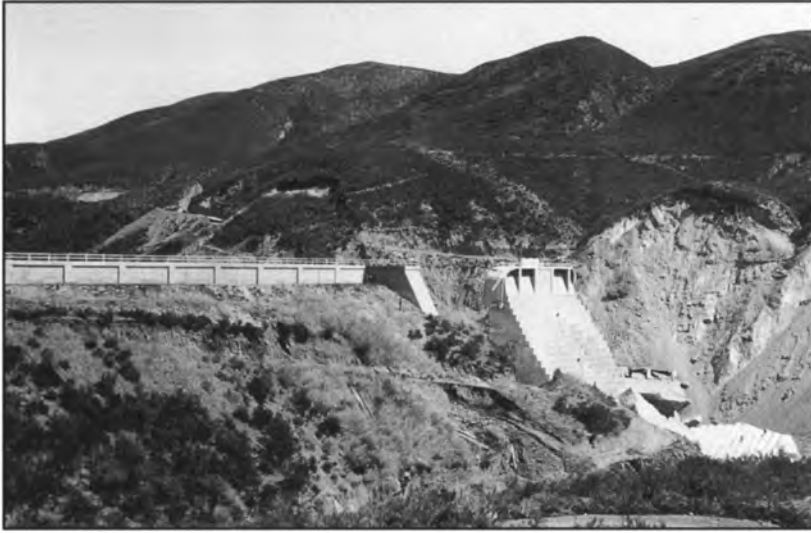
Figure 26 (upper) - View looking across side canyon just below right abutment, near position of Figure 1, just after the failure. Note how the vegetation scour line cannot even be seen, suggesting that the right abutment failed only after the reservoir had dropped at least 60 feet from the crest. Photo from the Huber Collection, University of California Water Resources Center Archives.
