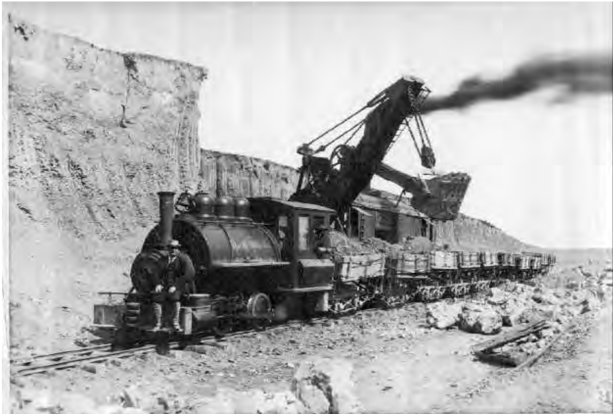
Figure 7 - Belle Fourche Dam Steam Shovel, Dinkey Locomotive, and Train of Side-Dump Cars in Borrow Pit
