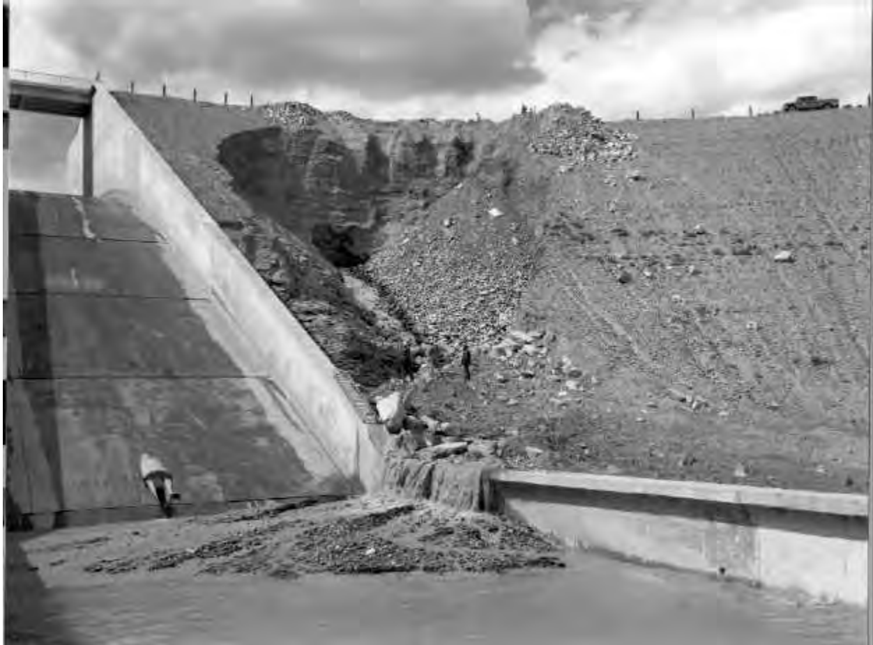
Figure 12 - Fontenelle Dam - Large Sinkhole on Downstream Slope
