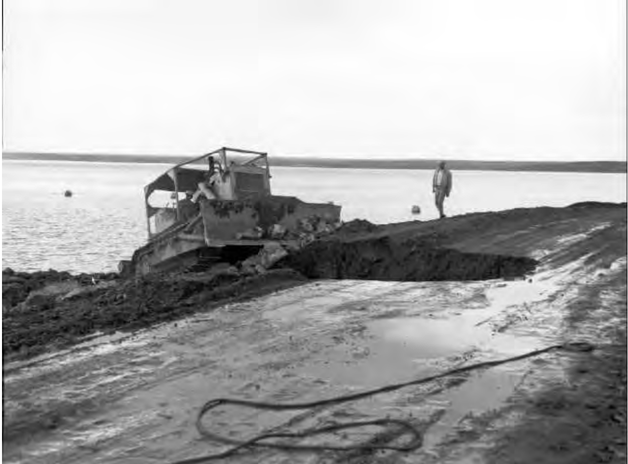
Figure 13 - Fontenelle Dam - Crest Sinkhole
