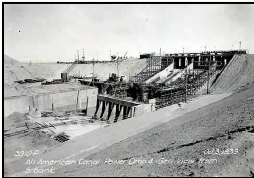
All American Canal Power Drop 4 –Gen View from S-Bank. Oct 3, 1939. Courtesy of Imperial County Department of Public Works.
