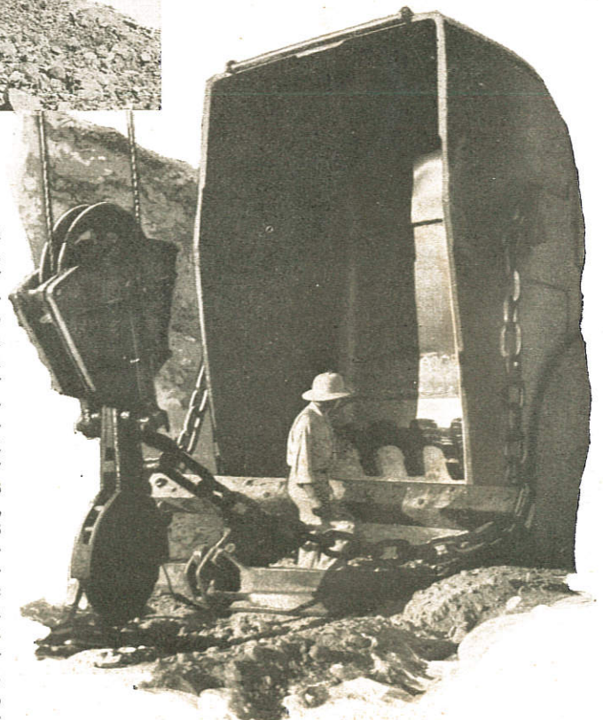
This is the big bucket of the drag-line, largest digger ever made. Shown here in the dumping position, it will hold an automobile
