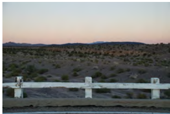
Figure 169 Existing timber rail with desert wash behind showing use of earthen berms to direct storm flows under the bridge.
