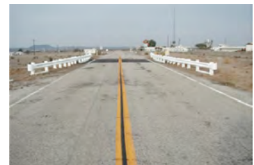
Figure 174 Existing 'W' shaped guardrail painted white (courtesy of San Bernardino County DPW); note post caps extend above the 'W' beam
